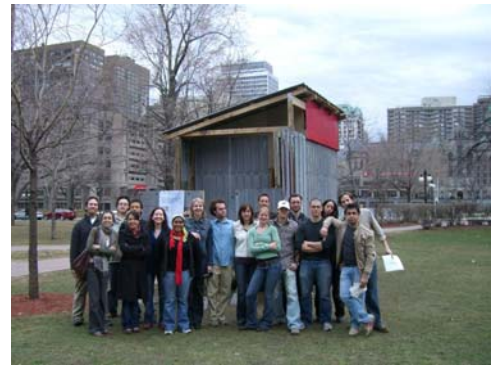
Fig. 9. Construction of an emergency shelter. In this exercise the students had to consider aspects of design, logistics and management (visible and invisible aspects) in order to build, in 3 days and with minimum tools, an affordable and environmentally-friendly solution for cold climates.
