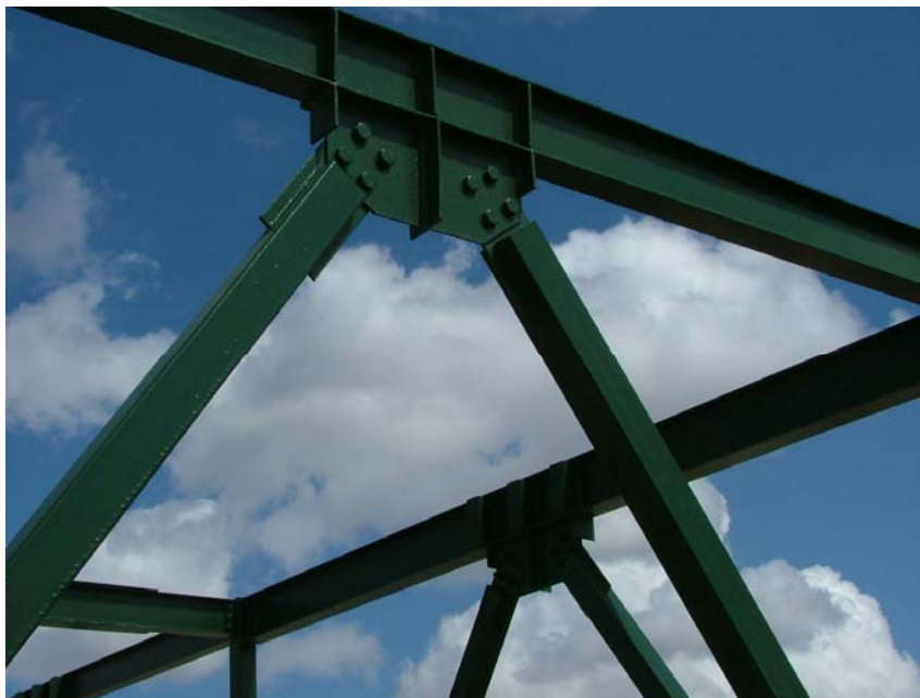
Figure 2: Detail of the HFIR's structure; posts and beams are connected by bolts and nuts
