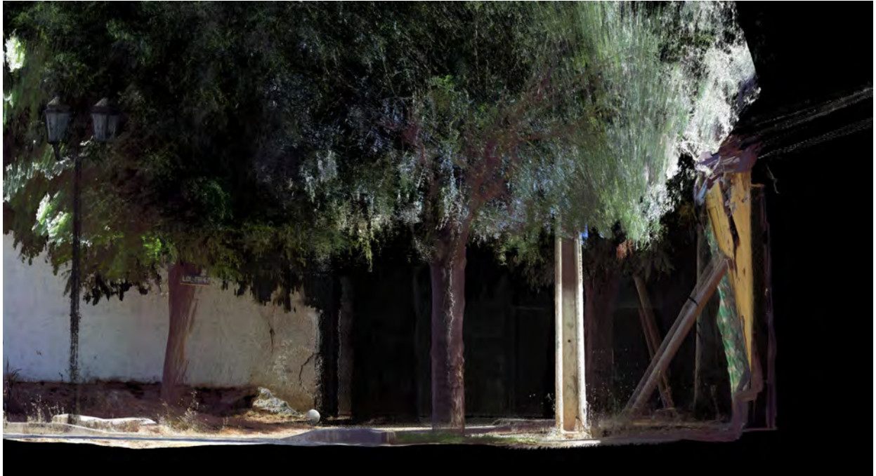
Figure 2. Section of a damaged dwelling in Lolol after the 2010 earthquake, where the deviation of the wall can be perceived. Rendered from the 3D laser scan data obtained in 2013. Source: B. Devilat.
