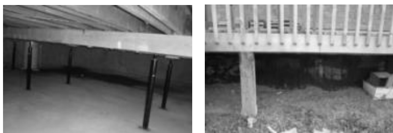
Figure 3: Adaptation mechanisms. Left: Strengthening in a house foundation. The original vertical support elements made of wood have been replaced by metallic ones resistant to moisture; Right: A newly built house rises from the ground level and does not have a basement, which is often vulnerable to floods.
