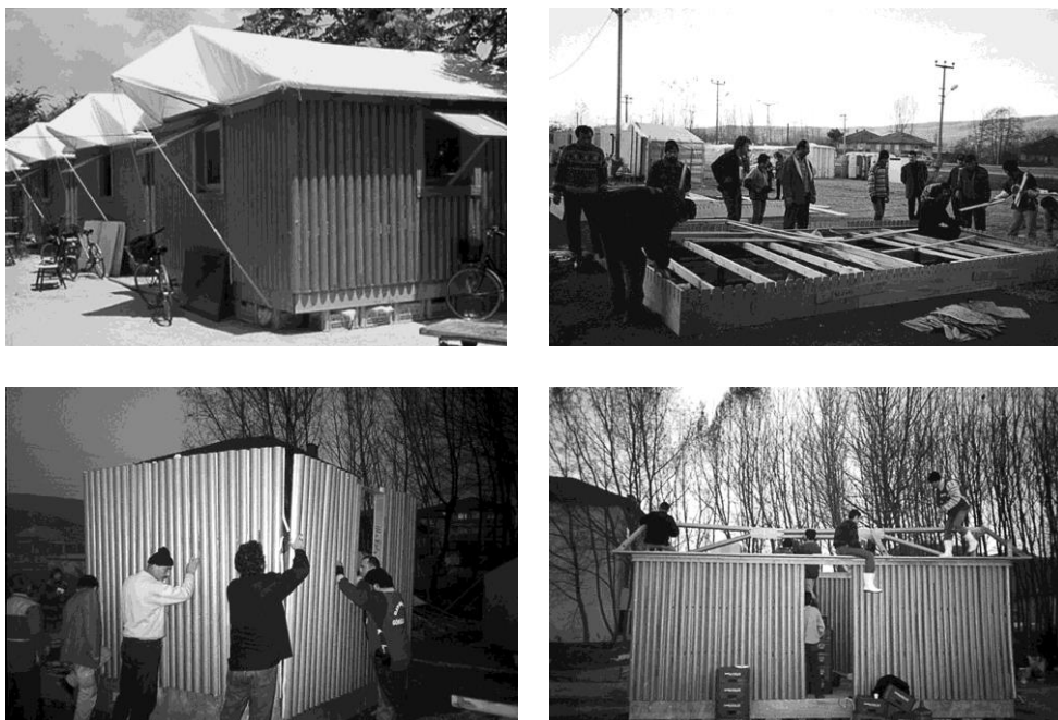
Figure 3: Paper Log Houses. Up-Left: Assembled units. Source: http://www.shigerubanarchitects.com ); Up-right, Bottom-Left and Bottom-Right: assembly works by local people. Source: https://archnet.org .
