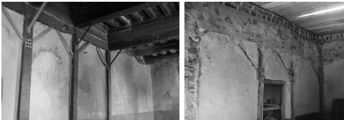
Figure 17: Left: Retrofitting technique used in Kharosa (C category village): wooden beams and posts tied through steel brackets; Right: Brackets introduced after the earthquake for retrofitting a traditional house have been removed by the owners to increase the height of the roof and replace Malwad with tin sheets. Source: Authors, 2011.
