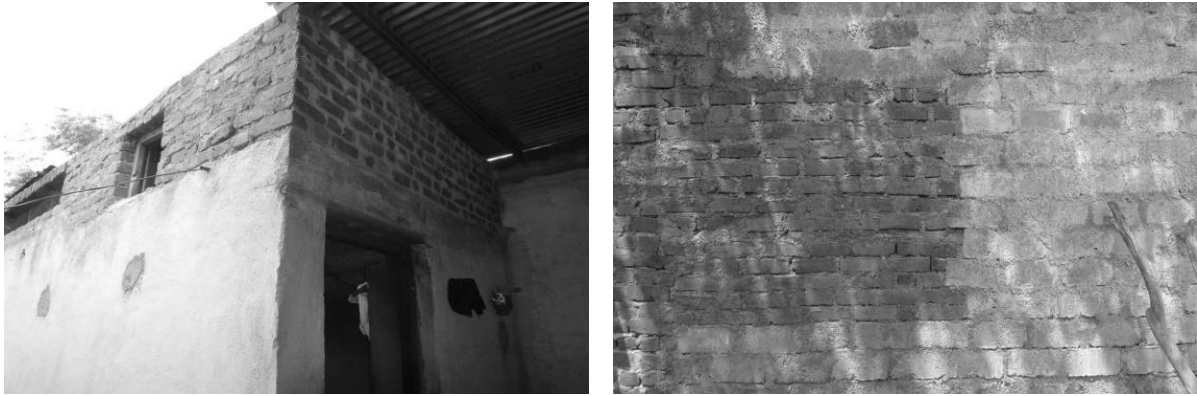
Figure 16: Left: High masonry walls lacking lintel bands in a Muslim farmer family house in Gubbal; Right: Wall made of hybrid materials in a Maratha farmer family, in Malkondji. Source: Authors, 2011.
