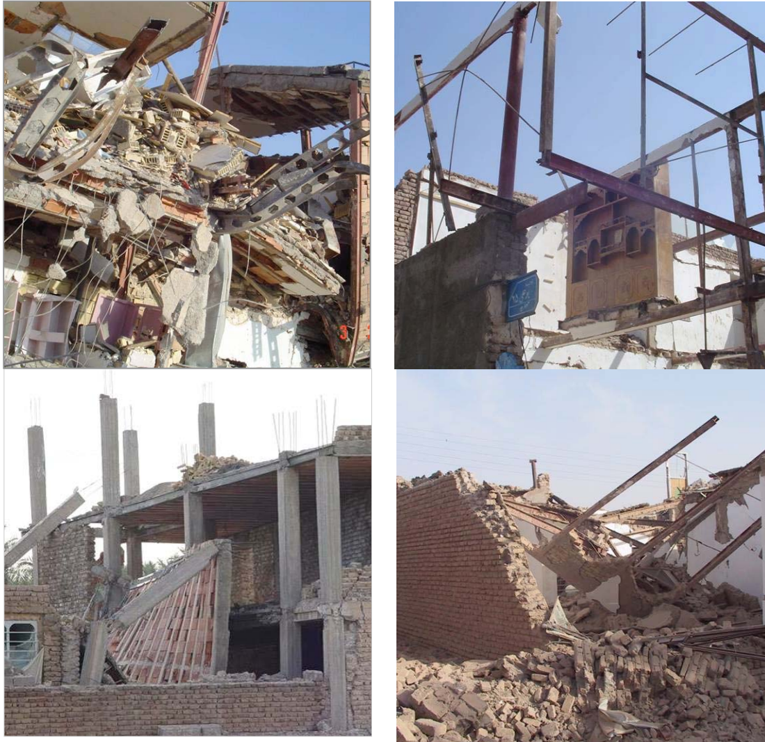
Fig. 4. Faulty building practice in Bam resulted in the high rate of casualties caused by the earthquake. (Photo source: HFIR).
